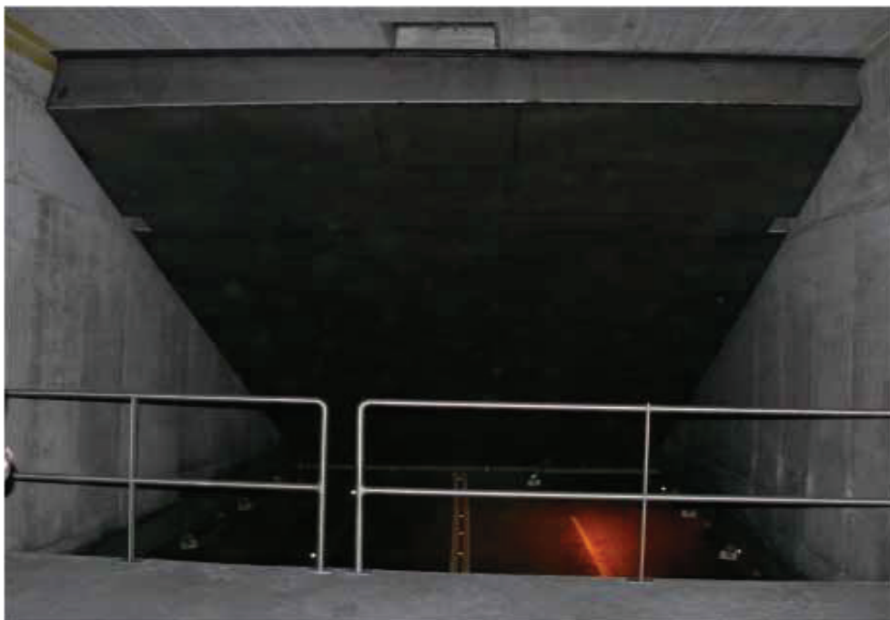
Figure 2: Flap gate, used for portal air extraction, open position
